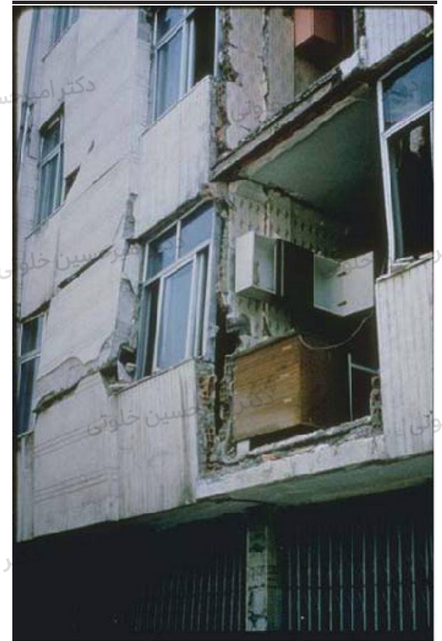
Manjil Earthquake – Northern Iran, June 21, 1990
